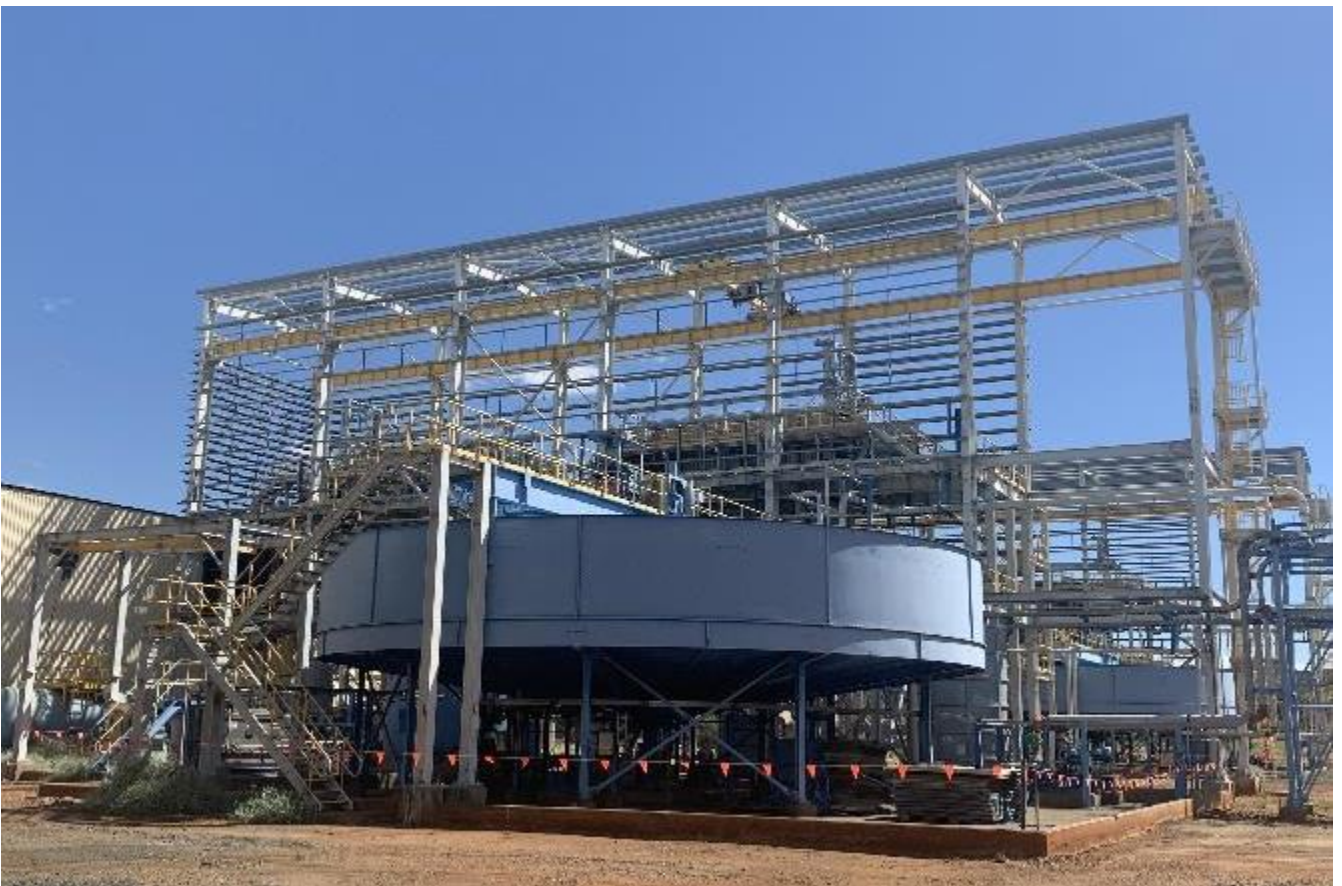
Figure 5: Tailings Filtration system including filter press (background) and thickener (foreground) that PNX is assessing for use at the Fountain Head project. The equipment would be transported and reconstructed at Fountain Head.
